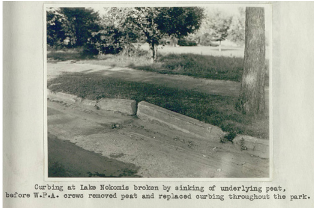
Figure 41 Broken Curbing. Curbing at Lake Nokomis was broken by the sinking of underlying peat and required WPA crews to remove the peat and replace the curbing. (Source: Minneapolis Board of Park Commissioners, 1939)
