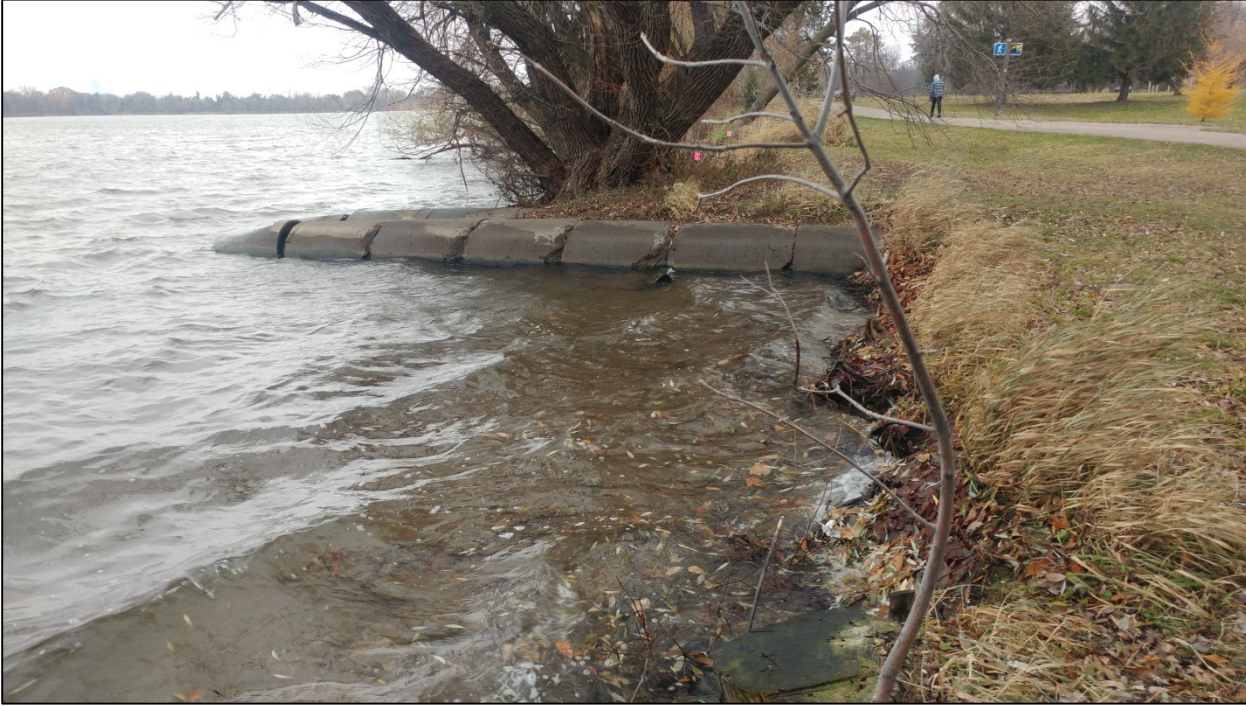
Photo 8. Existing Conditions – Erosion at east stormwater outfall.
