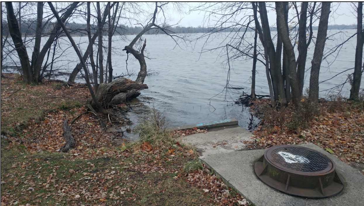
Photo 7. Existing Conditions – Erosion at north stormwater outfall.
