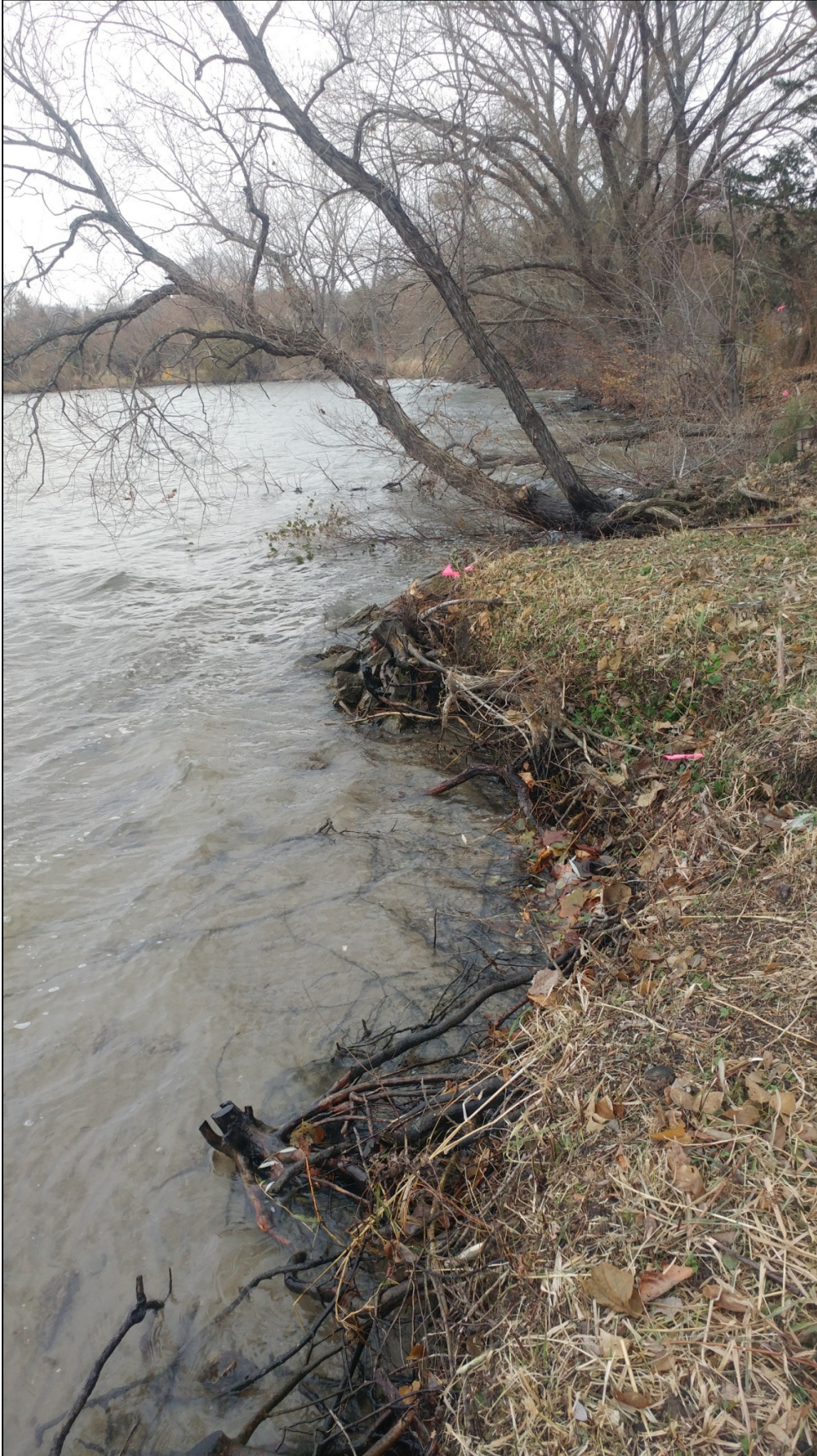
Photo 5. Existing Conditions – Erosion along lake’s east “Point”.
