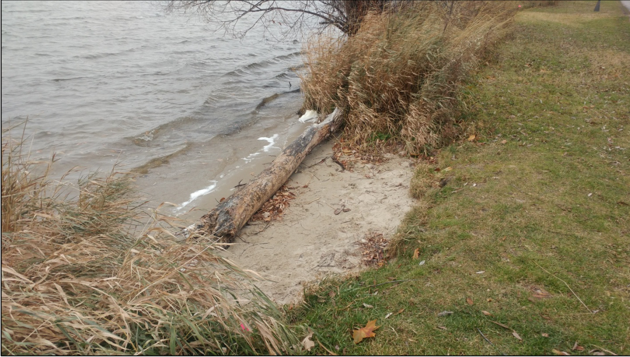
Photo 10. Existing Conditions – Minor erosion along lake’s east shoreline.
