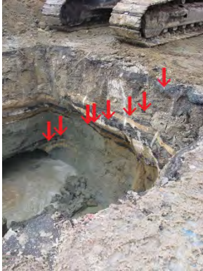
Excavation to fix exterior watermain break at existing mall. At least eight distinct repaving layers apparent extending about 6-feet below grade.
