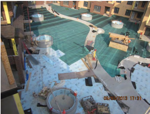
Under the charm – construction of waterproofing and drainage systems prior to adding soil media and plants on the green roof of the Folkestone Terrace West (fka, Superior Block). Photo courtesy of Adolfson & Peterson Construction.
