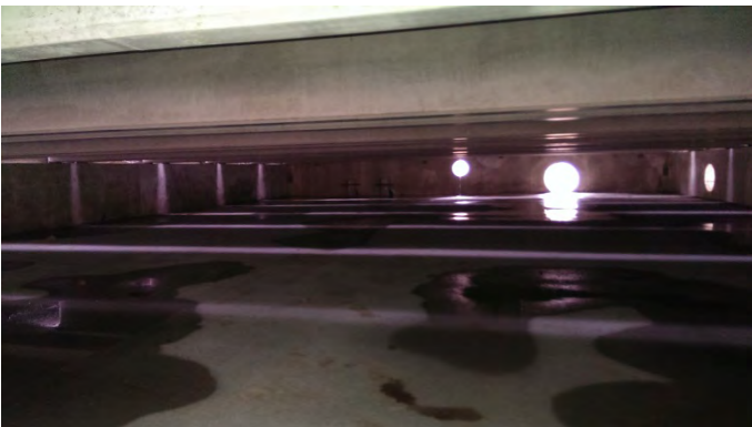
Looking south inside Engel Street detention vault during construction. Two large sun-filled round openings on right are for pending inlet pipes from project roof collection networks. Smaller higher opening on left is opening for eventual overlying street runoff collection pipe to route this dirtier runoff to the Mill Street filtration system.
