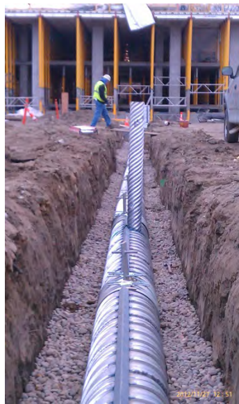
Trench drain risers and hanger connectors for storm sewer at The Promenade of Wayzata.
