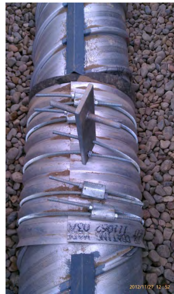
Hanger connector for storm sewer at The Promenade of Wayzata.
