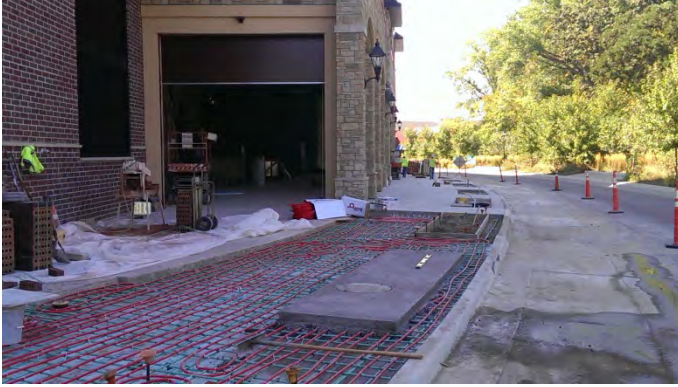
Hydronic snow-melt piping in walk by loading dock exit along Superior Boulevard at The Promenade of Wayzata.
