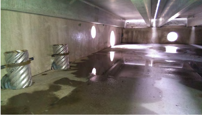
Two riser pipes for overflow of surficial portion of very infrequent storms rigidly connected to detention vault wall at south end of precast stormwater detention vault of Engel Street infiltration system (foreground). Riser rims set at 2.4-inch storm level, resulting in infiltration for 99% of annual rainfall for 5-acres of mostly impervious surfaces.
