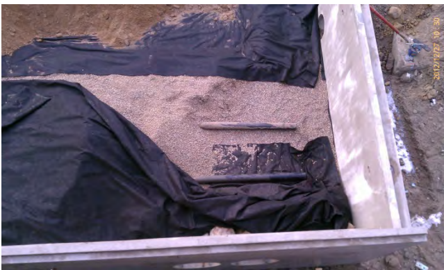
6-inch butt-fusion welded perforated drain tile in filter aggregate prior to slip-joint swivel connection to pending manifold pipe in Mill Street filtration basin.
