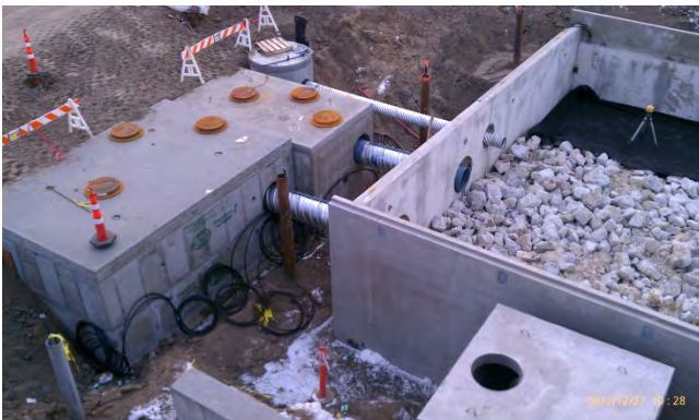
Large oil-grit swirl chambers over-pretreat boulevard runoff before discharging into the Mill Street filtration basin.
