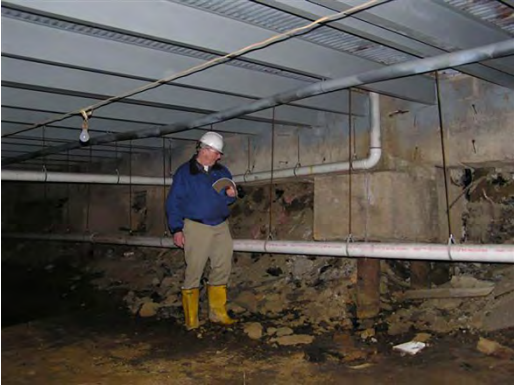
Inspector in “crawl space” below existing mall. Grade level is estimated to have settled about 5-feet since original mall construction in 1964. AET, Inc.
