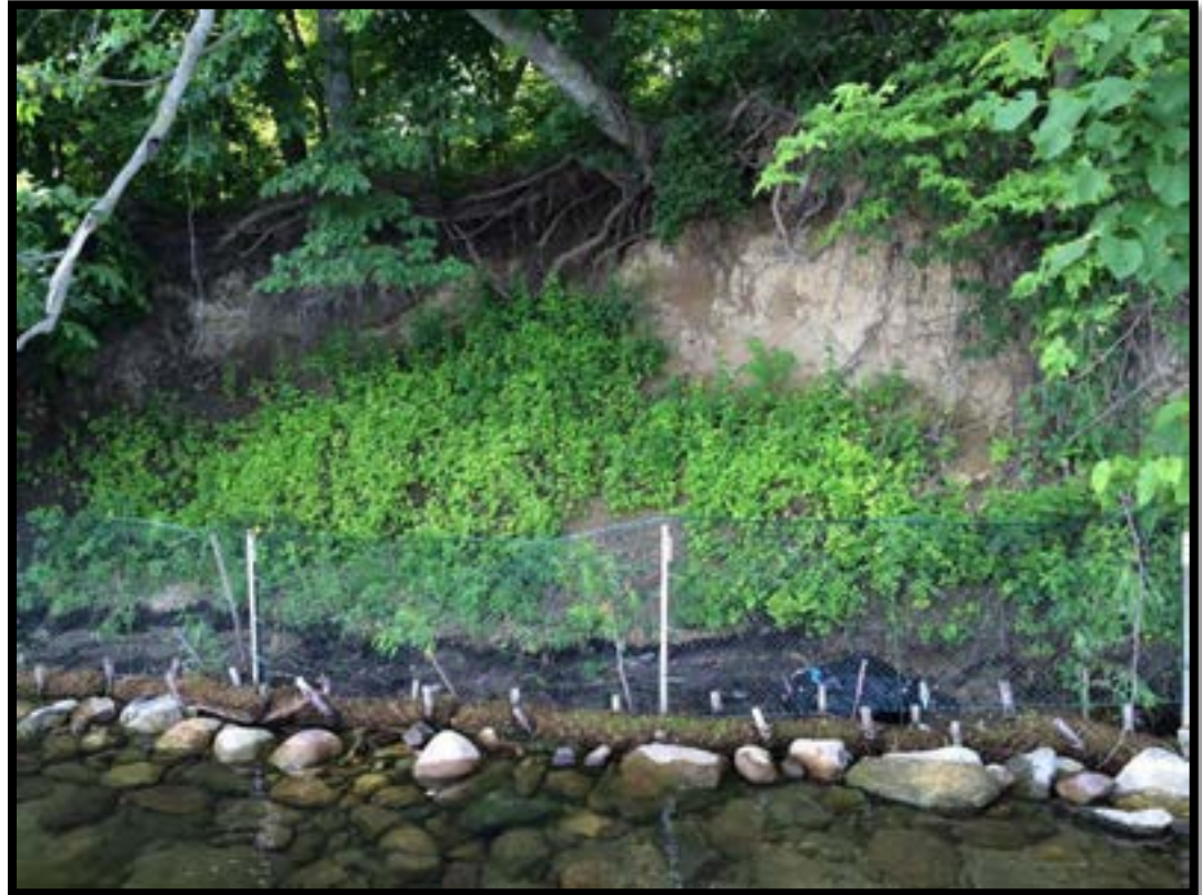
Topsoil erosion behind biologs at Big Island on July 14, 2014.
