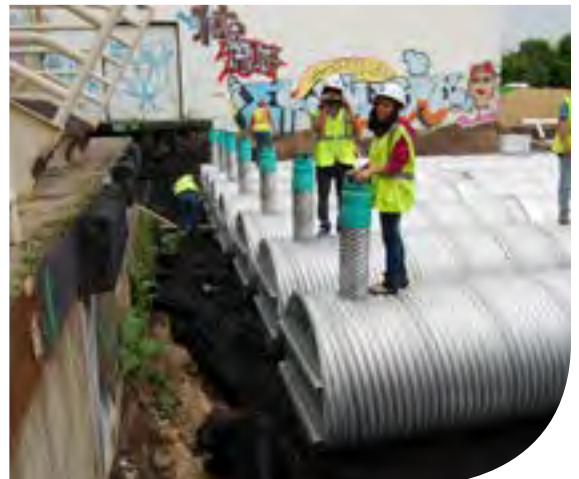
Underground stormwater treatment in Minneapolis
