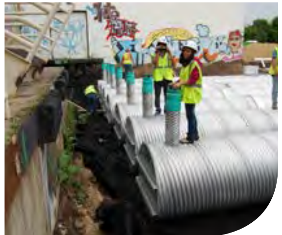
Underground stormwater treatment in Minneapolis
